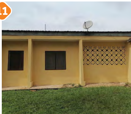
Facelift of OPD and provision of office furniture, suction machine for the Kranka Health Centre in Nkoranza North. ( Bono East Region )
